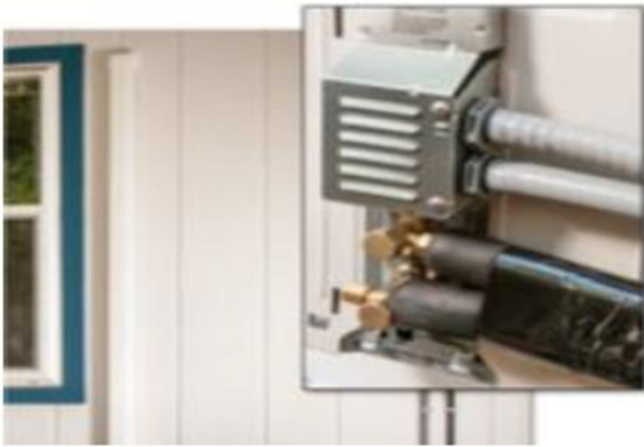
Line set properly insulated
