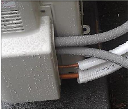
Line set not properly insulated
