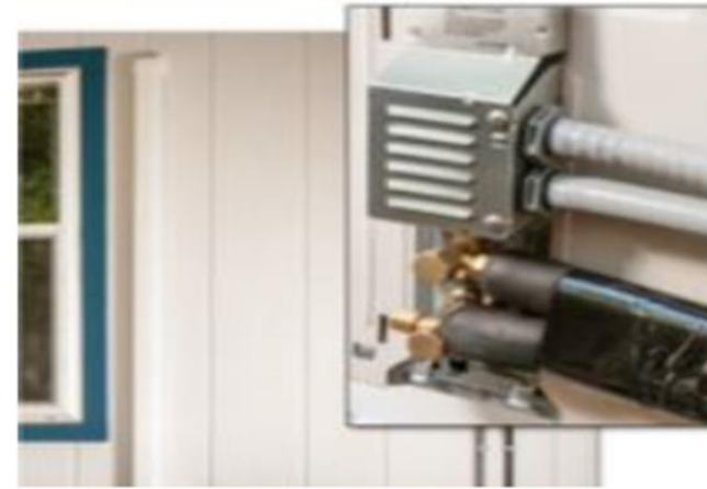
Line set properly insulated
