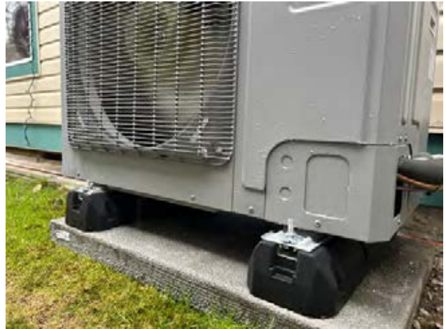
Figure 10 Heat Pump Installed on a Concrete Pad with Anti-Vibration Isolation Mounts
