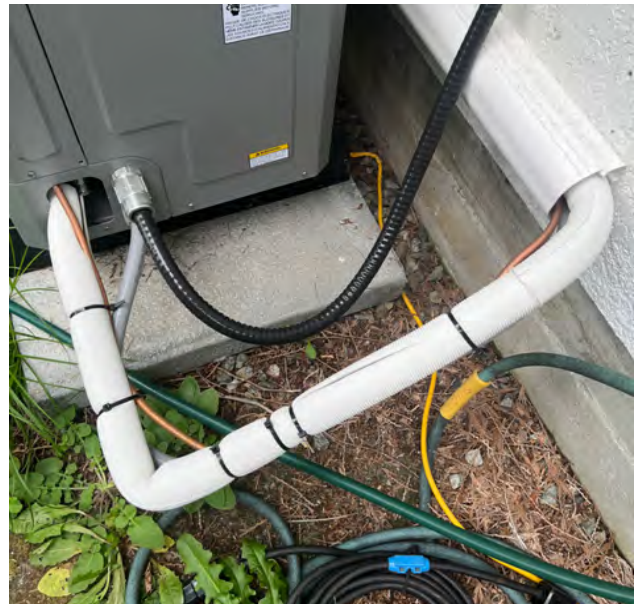
Figure 17 Insulated and UV Protected Refrigerant Lines
