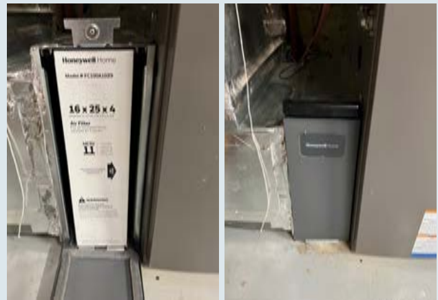
Figure 6 Filter Inside a Cabinet (left) and Sealed Cabinet (right)
