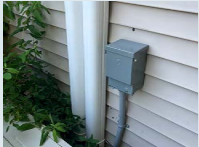
Figure 13 Protected Electrical Wiring and Disconnect
