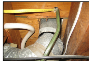
Disconnected duct, general leakage, and too small sizing means air isn't being delivered to the room
