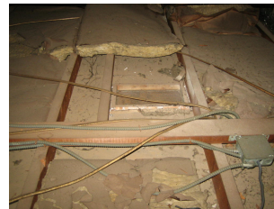
Missing/poor attic insulation makes it hard to keep heat in room in the winter and block heat out in the summer
